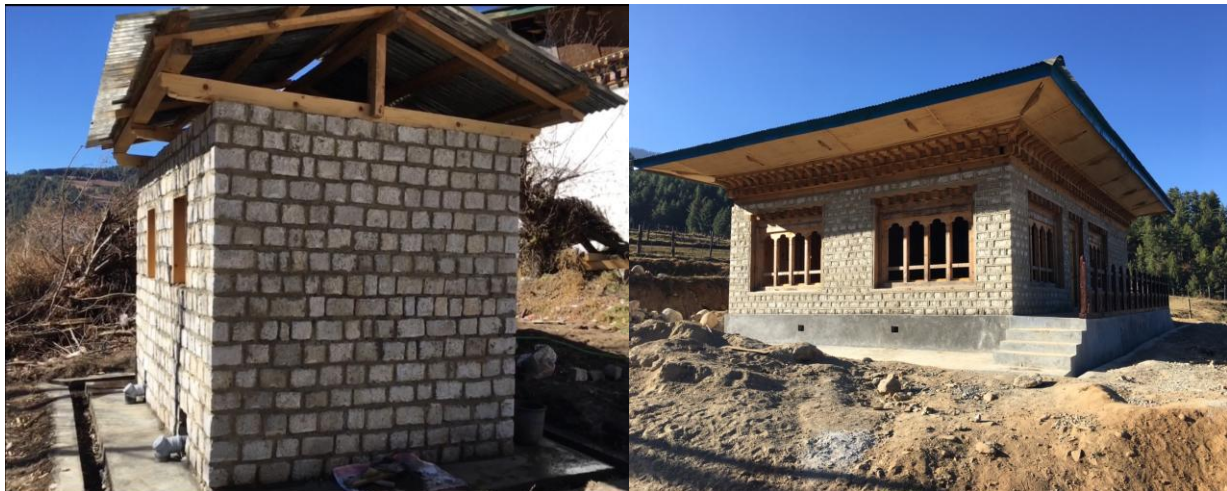
Toilet at the Gup's Office at Tang and Horse Farm Office at Bumthang constructed by TTI students, Chumey
